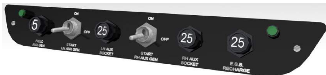
LH breakers rack: built-in generators field switches and system related breakers (panel type 2)
