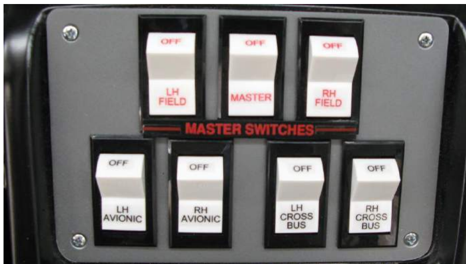
Central pedestal switches console
