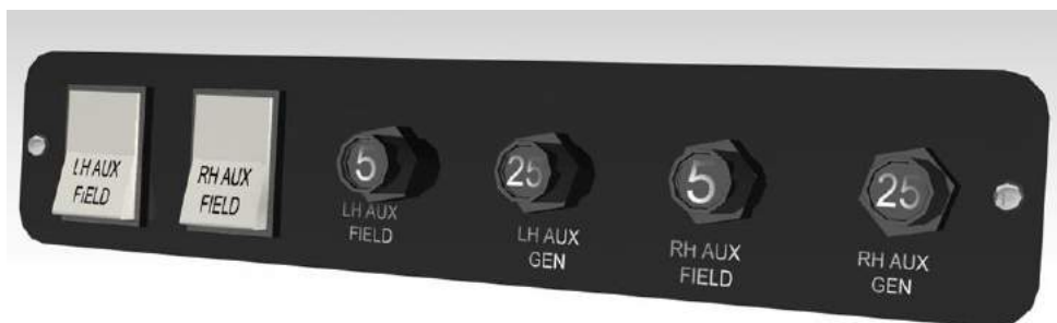
LH breakers rack: built-in generators field switches and system related breakers (panel type 1)
